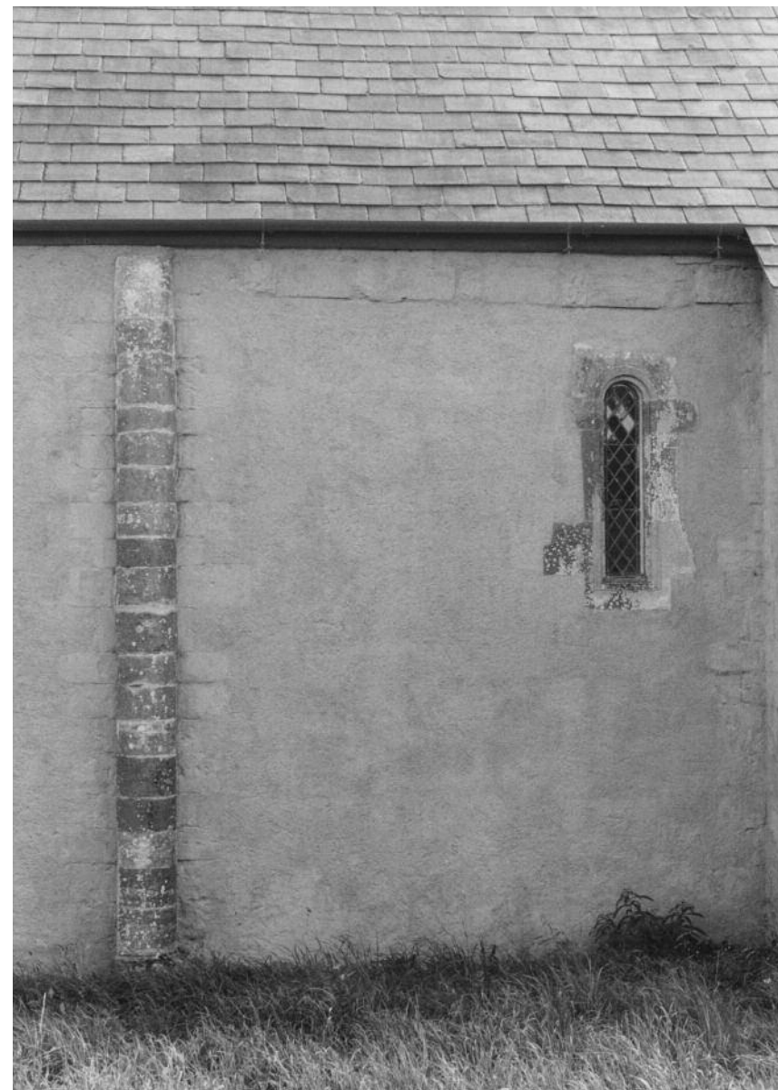
Exterior view of the north wall of the chancel, showing the 11th century buttress and lancet window, and the remains of the corbel table. (TOM MAYBERRY)
